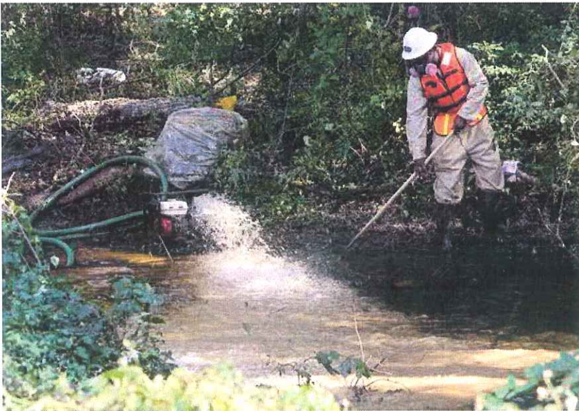
Workers clean up the 4,000 barrels of crude oil that spilled in Tete Bayou. Sunoco Logistics, operator of the Mid-Valley Pipeline, has responded with more than 250 personnel to the site to contain and recover the oil, which entered Tete Bayou but did not reach Caddo Lake. (Photo: Henrietta Wildsmith/The Times)
