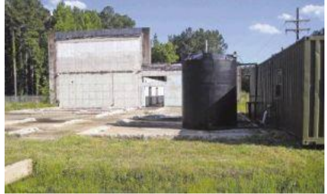
Chem Lab site treatment unit
