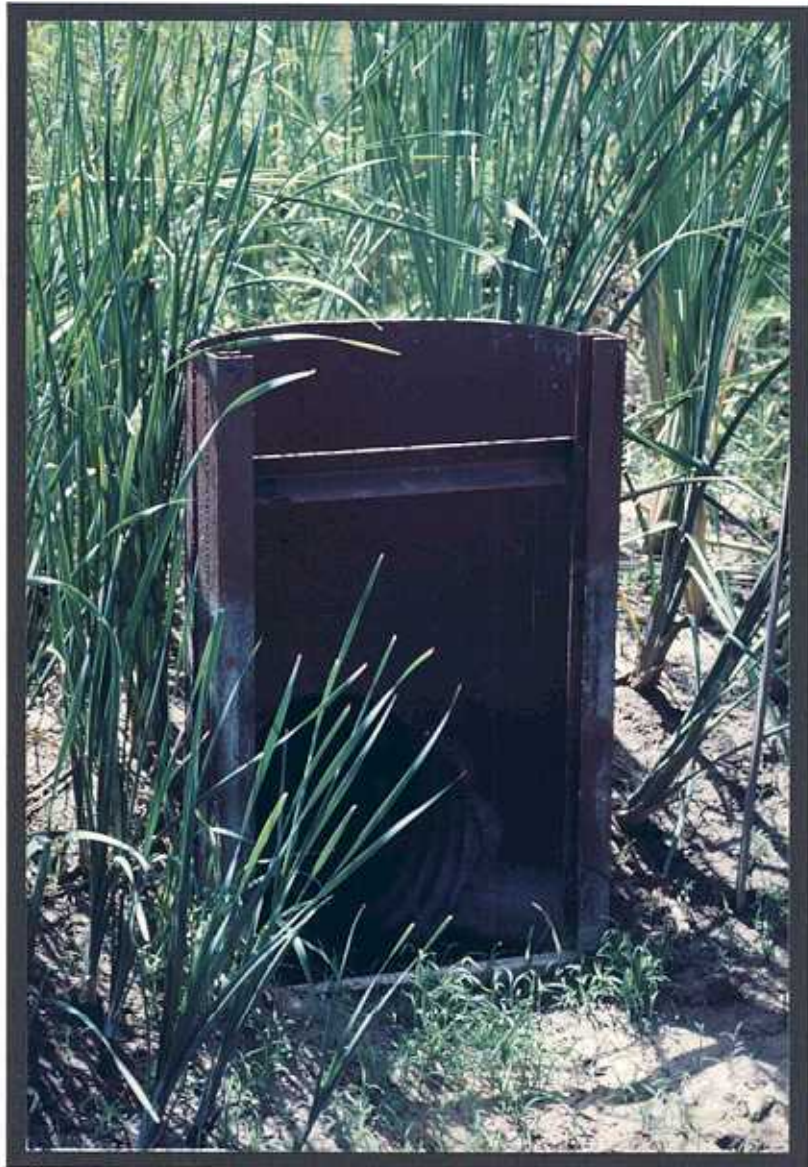
Figure 9. Flashboard riser used for water level management of restored wetlands.
